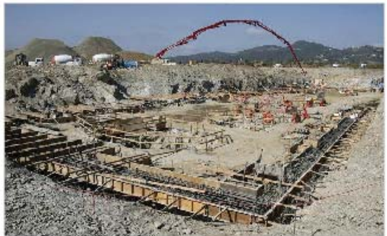
Construction workers make progress on the foundation and footing for Palomar Pomerado Health's new Escondido hospital Tuesday. (Photo by Don Boomer - Staff Photographer)
